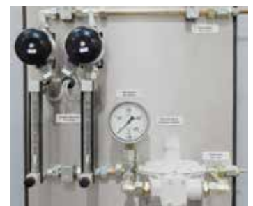
Gas supply system for non-flammable protective or reaction gases
